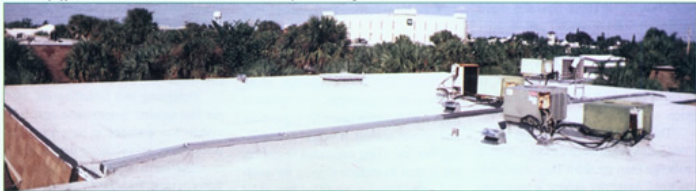
Dade County Approved aluminum hurricane stands were installed for roof top air conditioning units.
